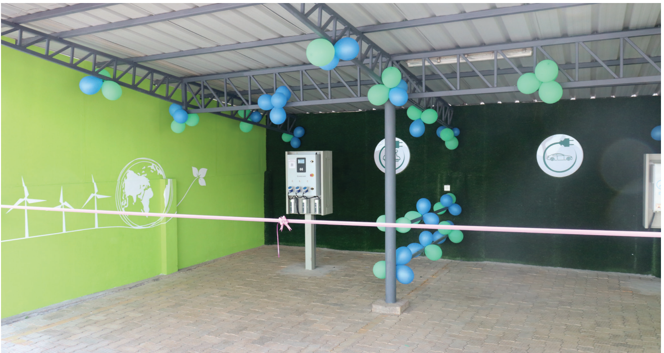
EV Charging Facility at Sahya
